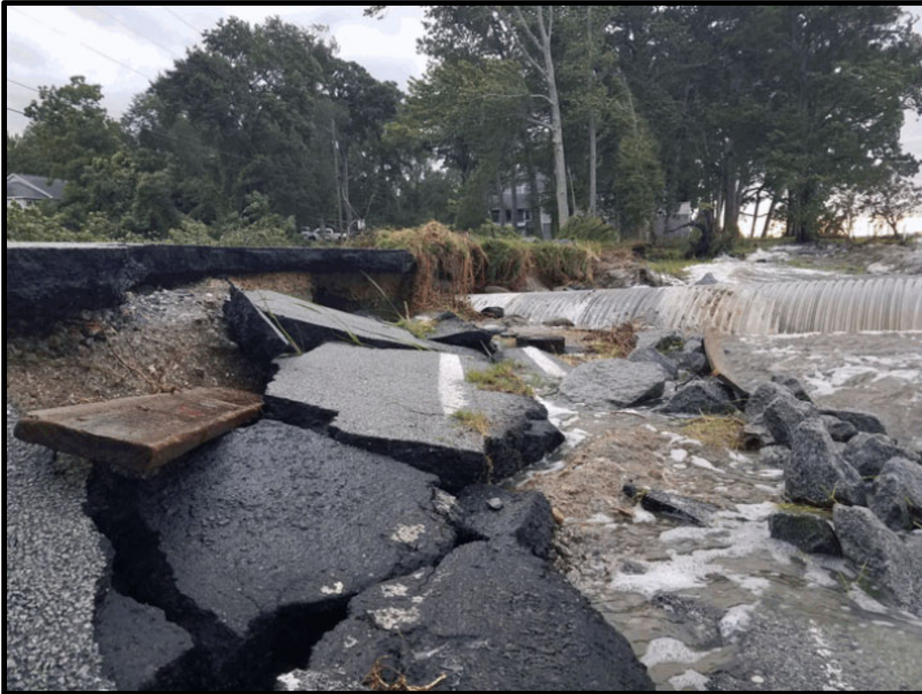
Figure 15. Storm surge damage in Bayview, NC. Image courtesy of North Carolina Department of Transportation.
