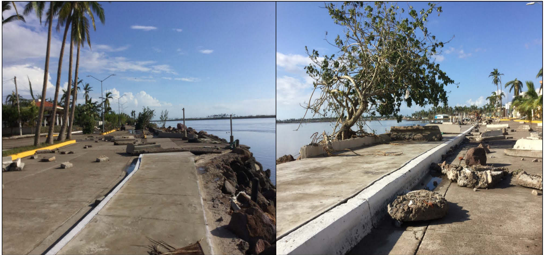
Figure 10. Damage to the seawall in the Malecón district of Teacapan, Mexico, where the eastern eyewall of Willa accompanied by the strongest winds and highest storm surge likely occurred – (left) viewing southeast along the coast and (right) viewing northwest along the coast. Images taken on 24 October 2018 courtesy of Josh Morgerman, iCyclone.com .
