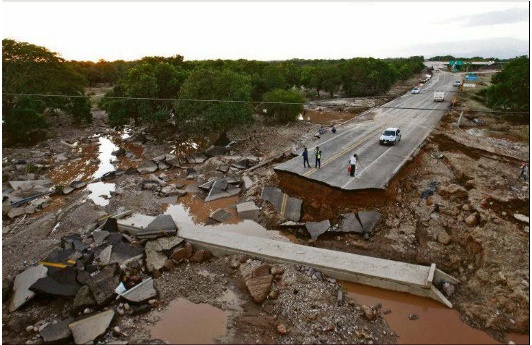
Figure 12. Bridge collapse and highway eroded over the Rio Acaponeta in Nariyat state, Mexico. Picture courtesy of Informador.mx .
